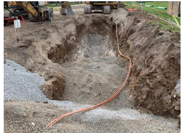
Trench in County Hwy II to extend sanitary sewer into the project site (8/31/2021)
